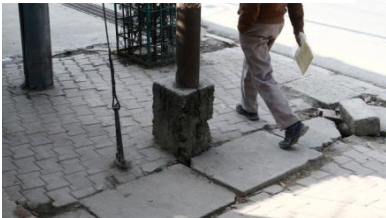
Figure 4: utilities on footpath Source: http://assetscdn.ekantipur.com/images/thekathmandupost/miscellaneous/photo-1-22122018075416.jpg
