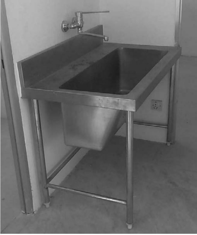
a. Stainless Steel Scrub Sink
